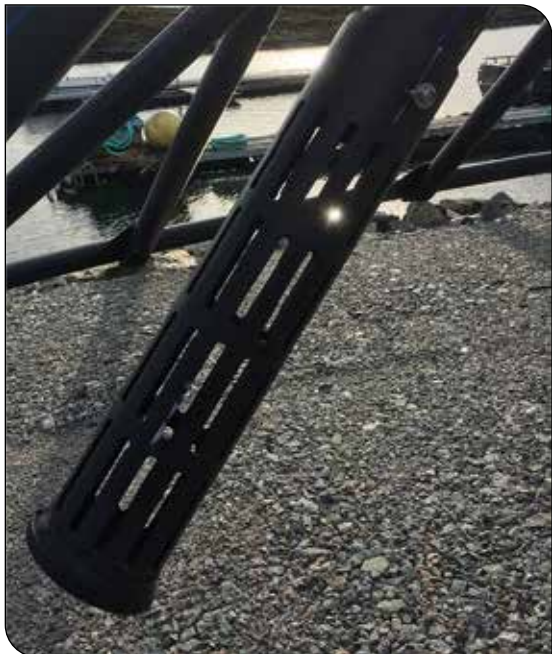
Illustration 2: Filter at water intake
